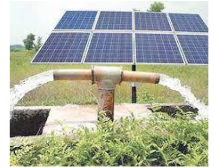
Rural Solar Water Pumping
