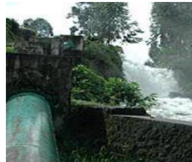
Hydropower IPPs (pipeline capacity of 45MW)
