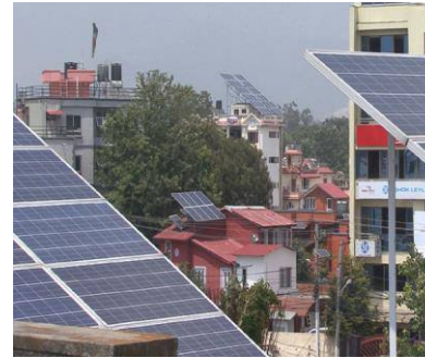
Distributed Rooftop Solar
